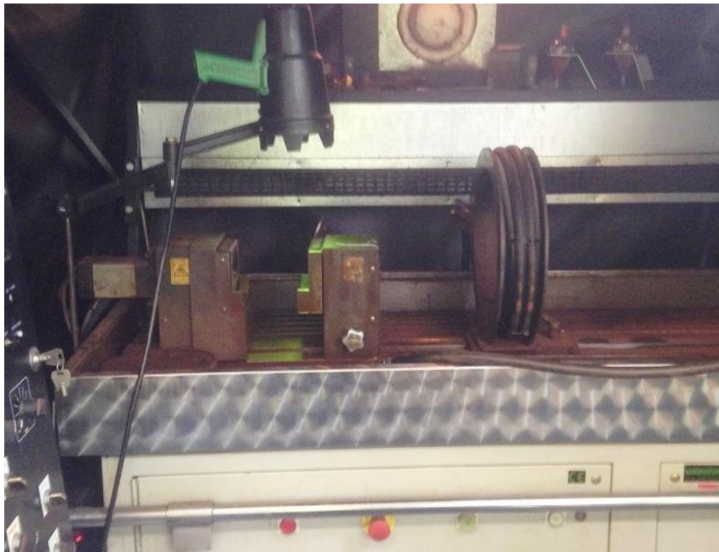
Figure 9 - Magnetic Particle Inspection (MPI) Unit.
