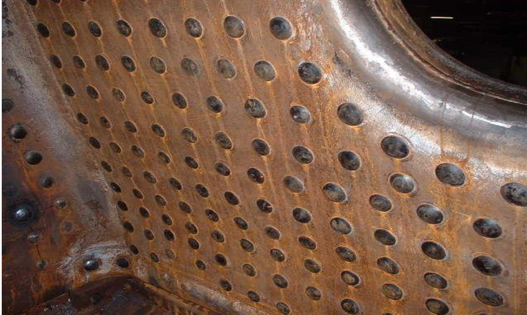
DEFECTS ASSOCIATED WITH LOCOMOTIVE BOILERS. BROKEN FIREBOX STAYS
