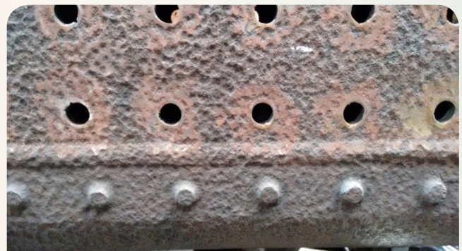
Figure 8. Exterior corrosion making ultrasonic coupling difficult
