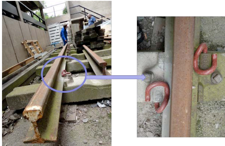
Figure 3. Pandrol PR clip system on an experimental section of rail at the University of Birmingham.
